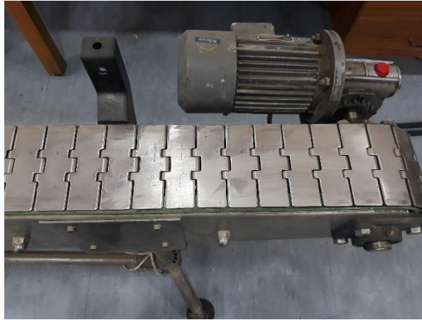
Figure 3: Conveyor belt system driven by 3-phase induction motor.
