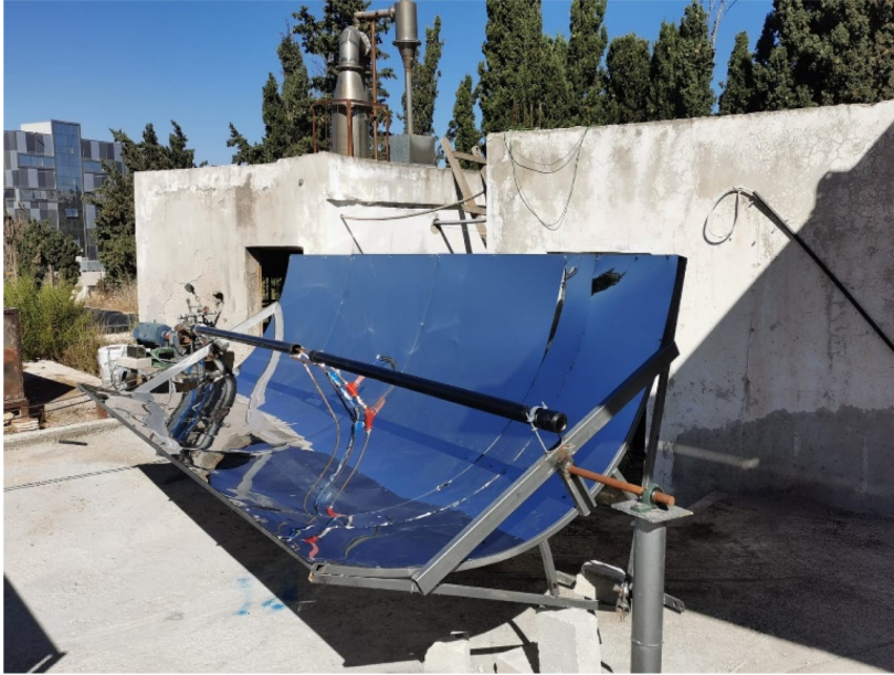
Figure 3. The constructed PTC system.
